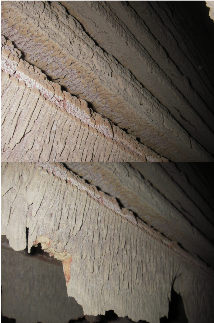
Fig. 5.3 Photography of deposits at a superheater in GKS plant
